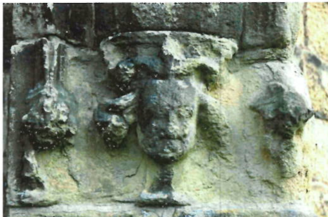
Photo 5.6: Erosion due to acidic rain, Eyam Church, UK. (Source: PA.)
